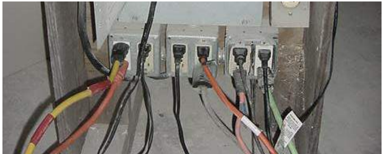
Common temporary set-up of electrical panel with GFCI outlets found on a construction site.
