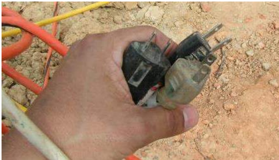
Never use extension cords that have broken or missing ground pins!
